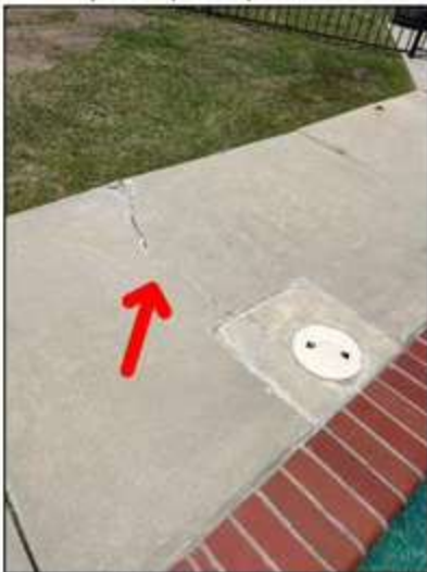
Pool deck has visible crack(s) at various areas (2), recommend further review and repair by licensed pool contractor to repair/replace pool concrete deck (2).
