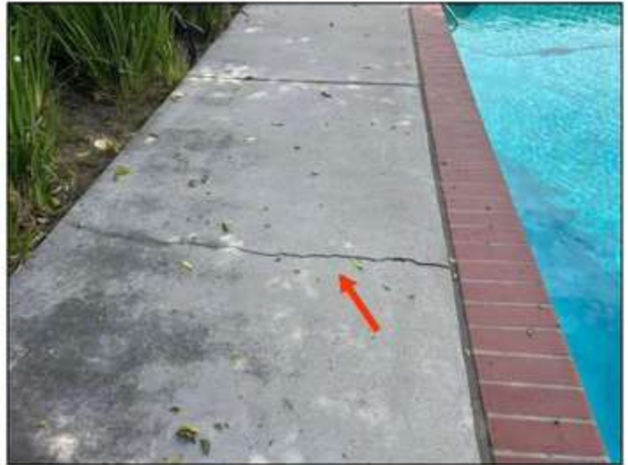
Pool deck has visible crack(s) at various areas (2), recommend further review and repair by licensed pool contractor to repair/replace pool concrete deck (2).
