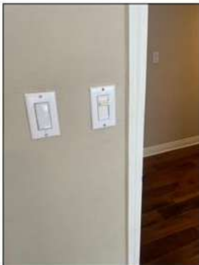
Bedroom #1 dimmer light switch on right side is non-function *(2).
