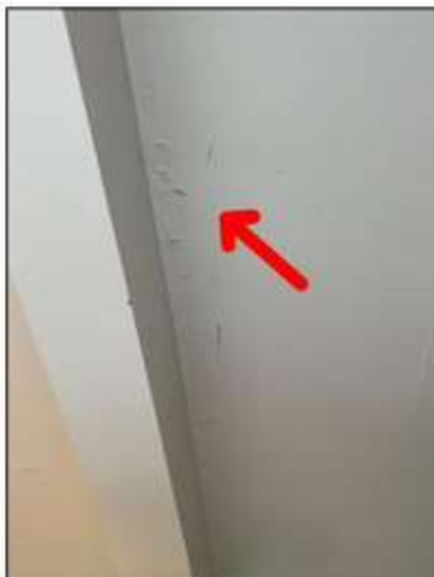
Chipped paint at kitchen ceiling *.
