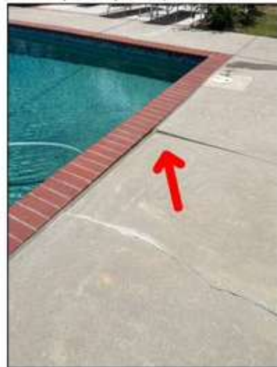
Concrete pool deck has settled area creating tripping hazard (4)*, recommend repair.
