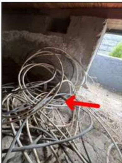
Excessive TV cable wire abandoned in foundation crawl space *, recommend removal as necessary.
