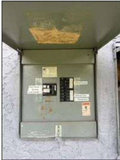
Sub electrical panel installed at exterior south side appears serviceable.
