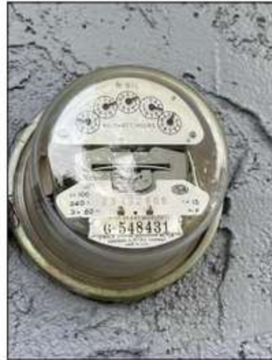
Electrical service main electrical panel Meter: 6- 100 amp meter installed, appears serviceable.
