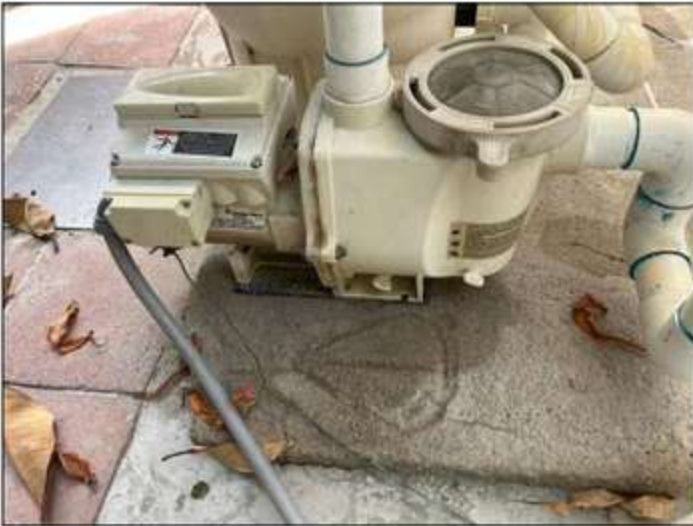
Pool has one pump installed, pool pump was tested, pool pump appears serviceable but may have other issue present. See notes below for other issues that may be present.
