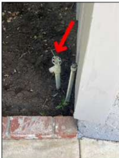
Exterior hose faucet is non-functional located at SW corner *. It appears that the property was re-piped with copper. This hose faucet may be abandoned.
