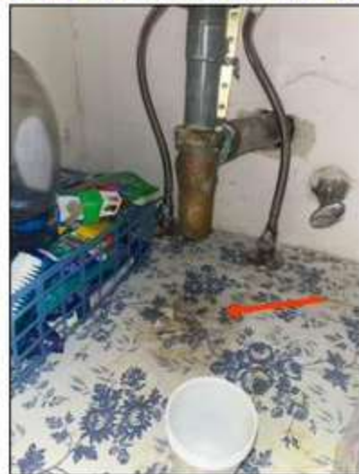
Bathroom (B) sink drain has active leak (2), moisture stain at base of kitchen counter. Recommend further review and repair by licensed plumber.
