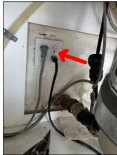
(gfc under sink) GFCI electrical outlets are required under kitchen sink (5)(2), recommend installing GFCI electrical outlets under kitchen sink as an upgrade. GFCI (Ground Fault Circuit Interrupter) outlets are required at kitchens to enhance electrical safety by reducing the risk of electric shock in wet environments. Even if a property was built before current standards mandated GFCI installation, upgrading to these outlets is crucial for ensuring safety and compliance with modern electrical codes. Retrofitting older properties with GFCI outlets not only protects occupants but also aligns the home with contemporary safety practices.
