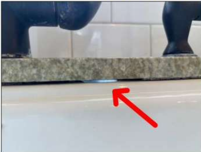
Undermount kitchen sink has visible gap at attachment under granite counter (2), this gap will allow moisture to leak under kitchen sink. Recommend repair as necessary.
