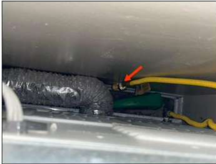
Gas supply valve to laundry area installed, appears serviceable.
