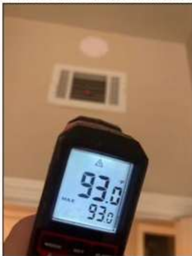
(normal temp) HVAC temperature on heating mode is 93°F, appears serviceable.
