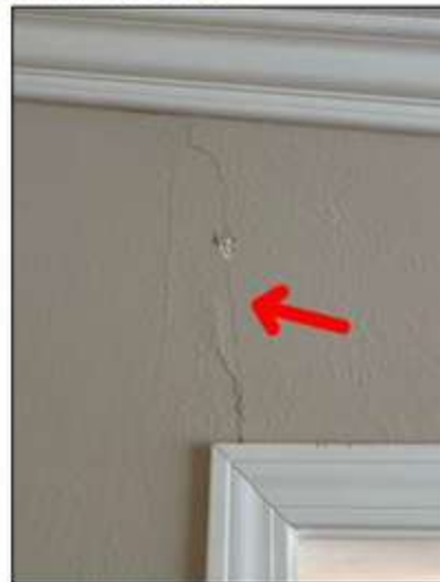
Living room Wall is cracked located on south side at door header (2).
