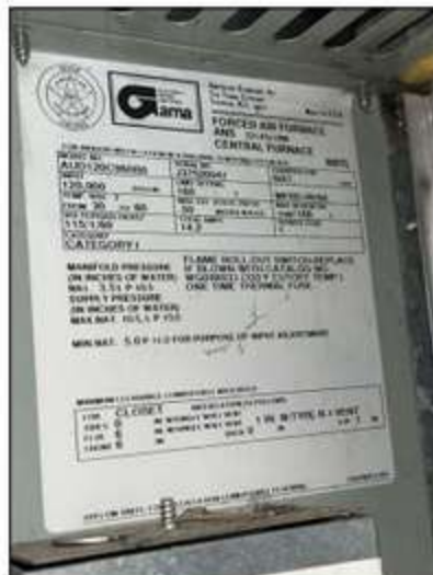
HVAC furnace MFG date: 1994
