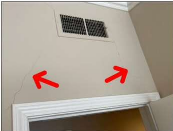
Bedroom #1 interior door header is cracked *(2).
