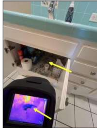
Bathroom (B) sink drain has active leak (2), moisture stain at base of kitchen counter. Recommend further review and repair by licensed plumber. The thermal imaging camera was used to inspect area which detected active leak.
