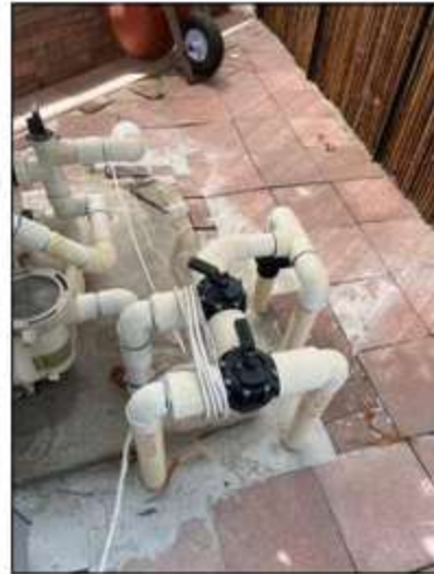
Pool has one pump installed, pool pump was tested, pool pump appears serviceable but may have other issue present. See notes below for other issues that may be present.
