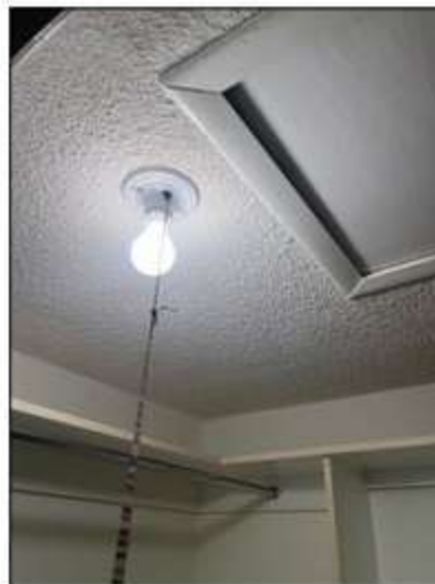
Bedroom #2 closet has a temporary ceramic light fixture without a proper cover install installed *(5). Recommend installing a modern light fixture as an upgrade.
