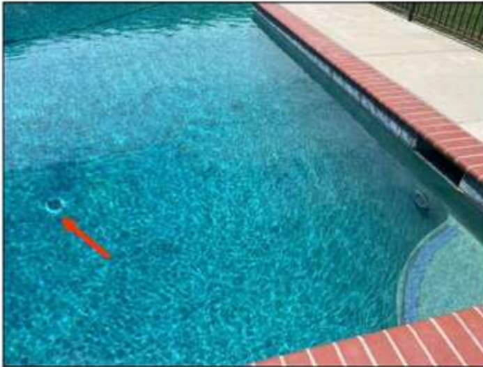
(missing proper Cover) Pool drain at the deep end is missing proper anti-vortex cover (5), proper pool drain covers are required to be installed as a safety upgrade. Current standards require two separate anti-vortex pool drain covers.
