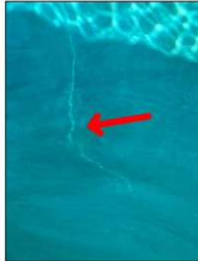
Pool body plaster has a visible crack/fracture in the middle section of the pool plaster, in addition a water hose placed inside the water suggests an active effort to compensate for water loss (2). The pool appears to be leaking, recommend further review repair by licensed pool contractor.
