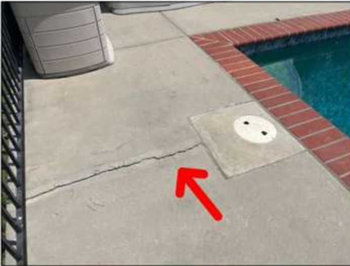
Pool deck has visible crack(s) at various areas (2), recommend further review and repair by licensed pool contractor to repair/replace pool concrete deck (2).
