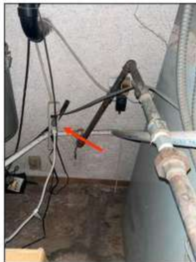
The HVAC furnace electrical cord is installed on an extension cord *(2), it is not recommended to connect the HVAC system on an extension cord. Recommend installing electrical outlet at this area to service HVAC furnace as required by current standards.
