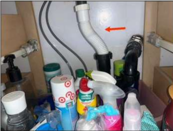
(flex drain A) Bathroom (A) sink drain has a flex extension form fit drain installed which is not approved in most areas (2), recommend further review and repair by licensed plumber.
