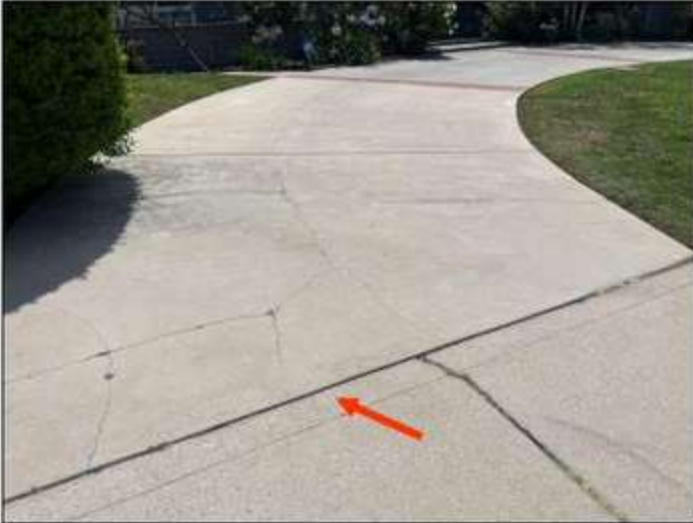
(trip hazard city) Driveway is settled/lifted at city sidewalk creating trip hazard *(4).
