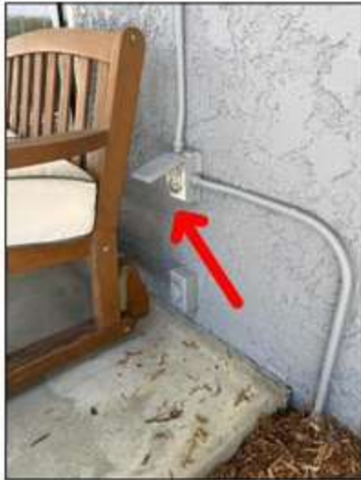
(ext gfci trip) Exterior GFCI located at rear patio did not shut off/trip when tested (4)(2), safety hazard. Recommend further review and repair by licensed electrical contractor. Location: Rear patio
