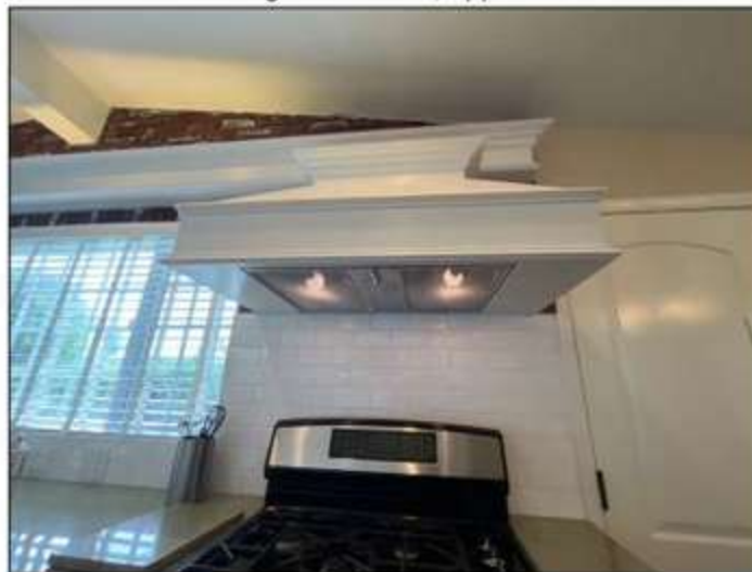
Kitchen exhaust vent hood installed, appears serviceable.
