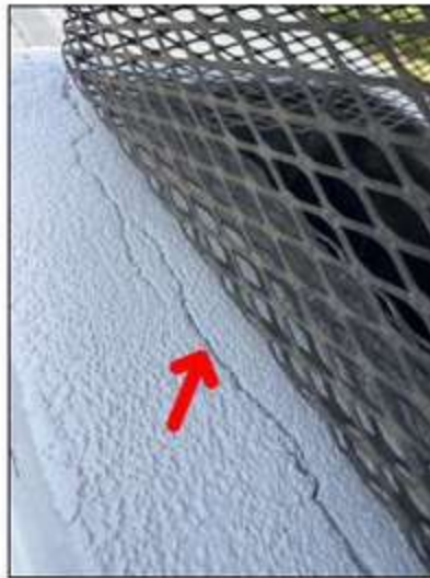
(crack crown) Chimney rain masonry cap/crown is cracked which will allow water to enter into inner chimney brick and mortar which prematurely age chimney deteriorating structure (2), recommend repair.
