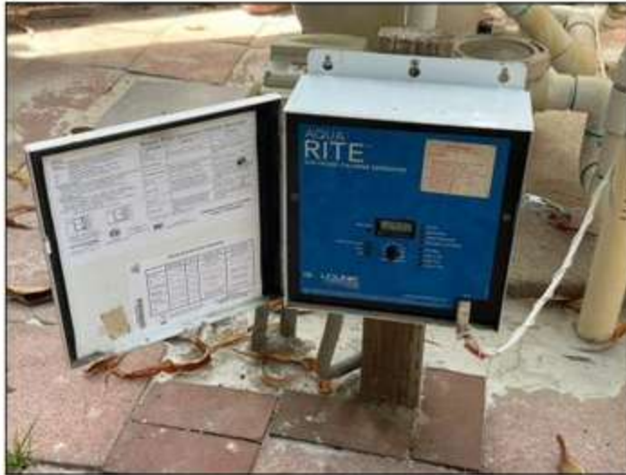
Who equipment chlorinator installed, appear serviceable.
