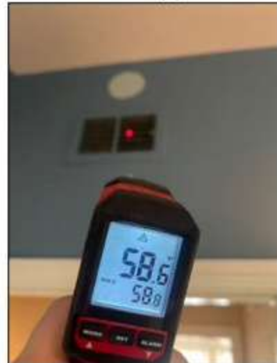
(temp) HVAC temperature on cooling mode was 58°F, appears serviceable.
