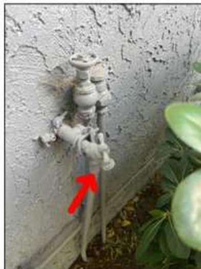
Exterior rear hose faucet is non-function *(2).
