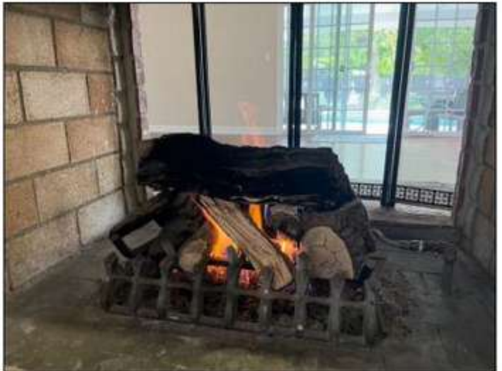
Fireplace (A) gas shut off valve installed, appears serviceable.
