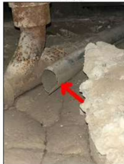
The whole house vacuum system piping/ducting in foundation crawlspace is nonfunctional and cracked at various areas *. Recommend re-installing piping/ducting if you would like to use whole house vacuum. Whole house vacuum was not tested *.
