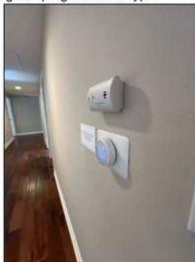
Thermostat located at main hallway.
