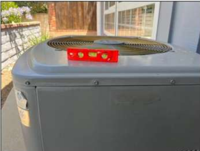
(not level) HVAC compressor is not level *(2), compressor fan requires level platform for proper function of compressor components. Having a compressor that is not level will prematurely wear compressor components. Recommend repair.
