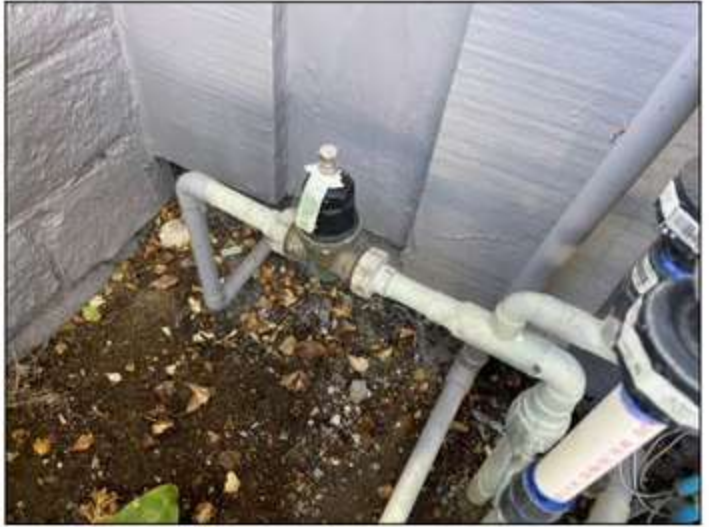
Main water supply pipe pressure regulator installed, appears serviceable.
