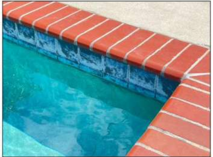
Pool tile is stained *, recommend repair/cleaning tile as necessary *.
