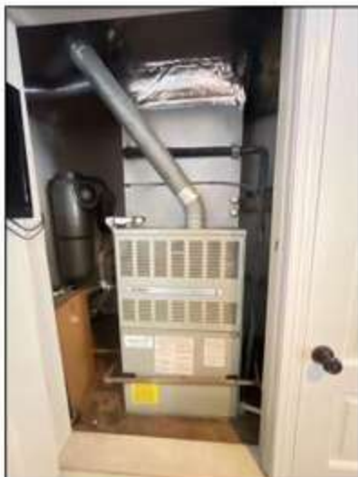
HVAC furnace installed is functional, but may have other issues present. See notes below for further information.
