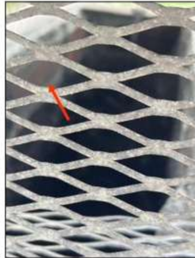
(no flue liner) Chimney did not have a flue liner as required by current standards (5)(4), the property was built before current safety standards, recommend installing flue liner as a safety upgrade (5).
