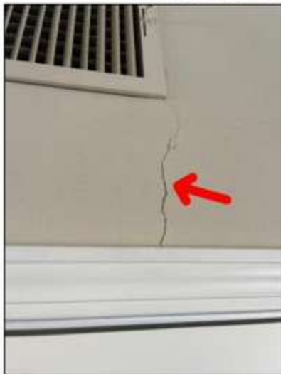
Main hallway closet Wall is cracked over door header *(2).
