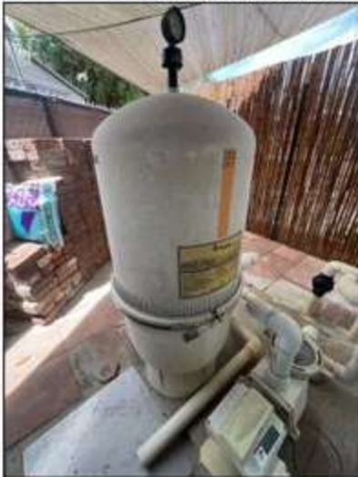
Diamtomaceous earth filter installed, appears serviceable. Interior of filter canister was not opened/inspected *. Recommend having Pool contractor clean and service filter as a preventative maintenance measure or ask home owner when last time pool was serviced.
