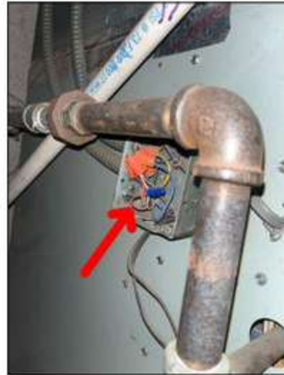
Electrical junction box located at HVAC furnace area is missing cover *.
